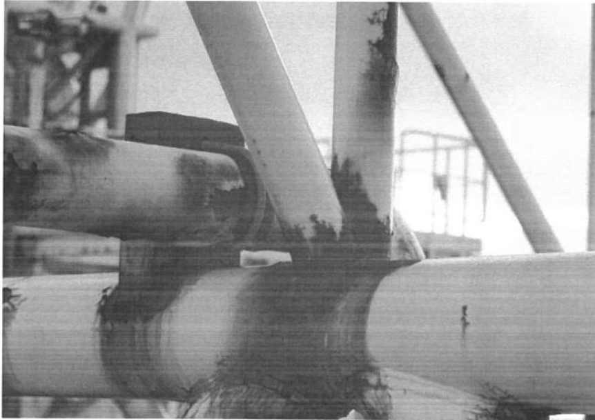
A typical example of corrosion taken on a North Sea platform
